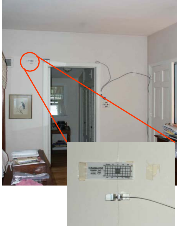
Figure 2.7 Wall view and detail photographs of Cracks 1 (top) and 3 (bottom) with sensors
